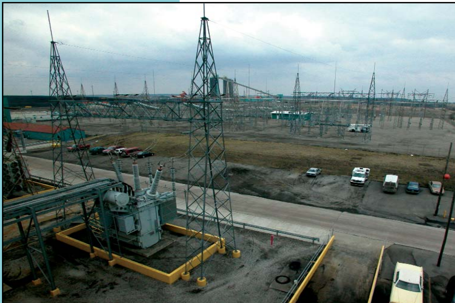
Power lines connecting to the Kansas City Power & Light facility
