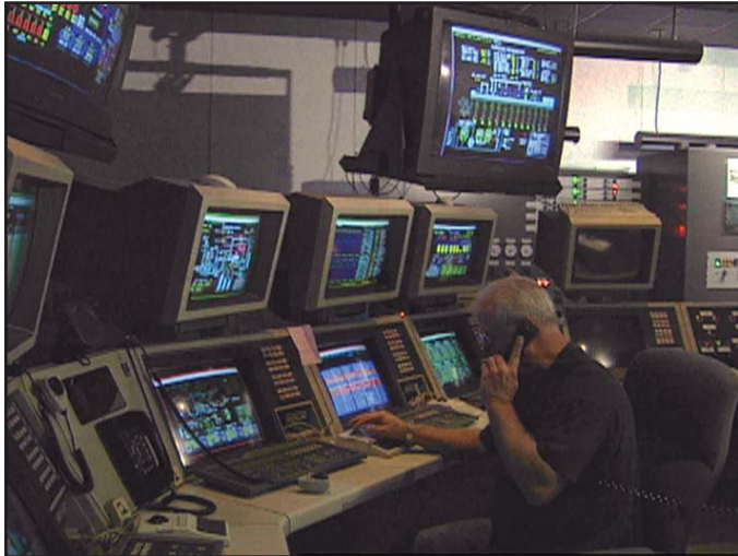
An operator monitors plant activity in KCP&L's control room.
