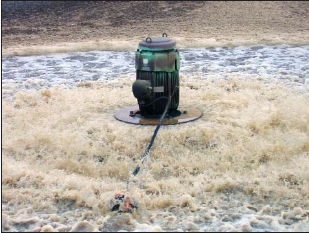
Close-up View of Clarifier
